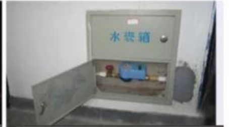
WATER METER BOX
