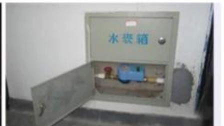
WATER METER BOX
