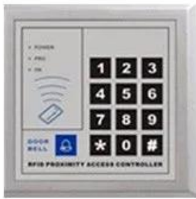
access control system
