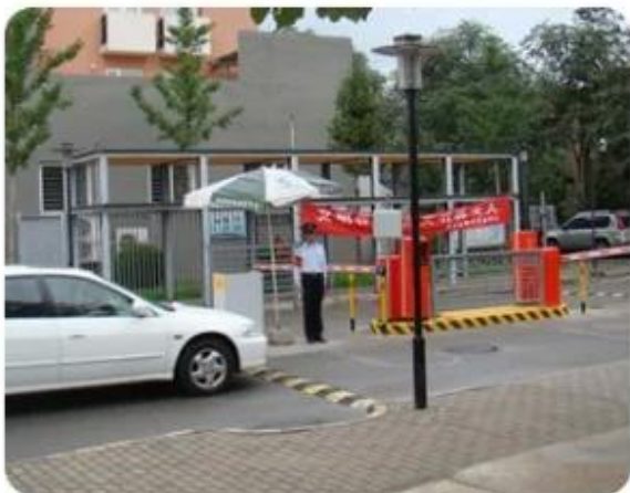
Parking lot vehicle access control system
