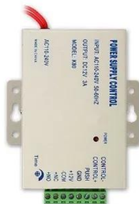
Access Power Supply
