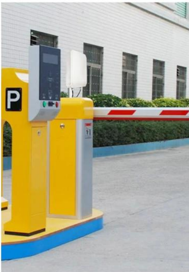
Vehicle Access Control
