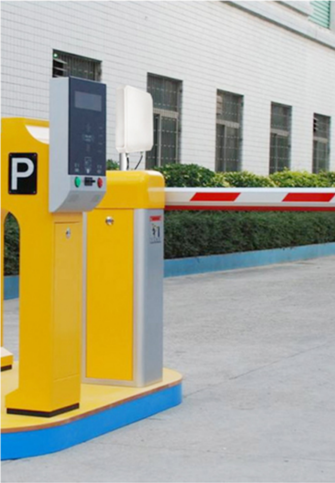
Vehicle Access Control
