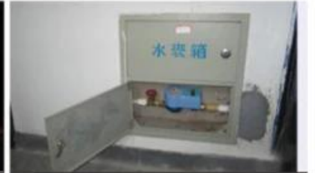
WATER METER BOX
