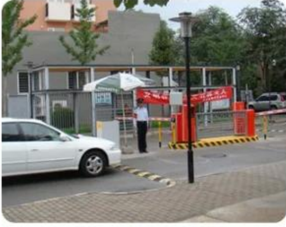
Parking lot vehicle access control system
